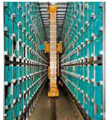
Storage & retrieval machine (SRM)
