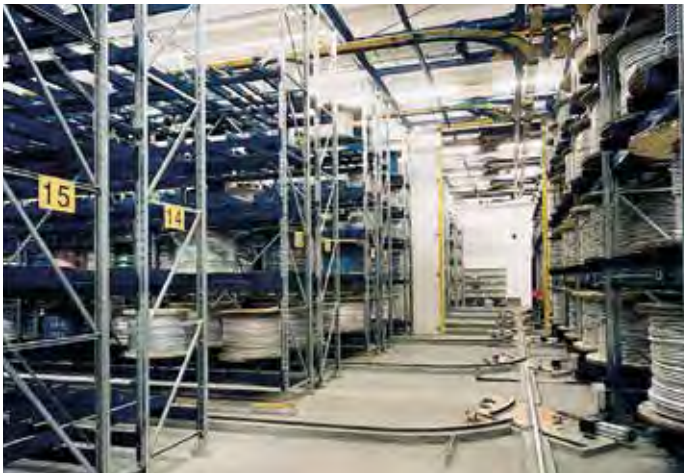
Aisle-independent stacker crane
