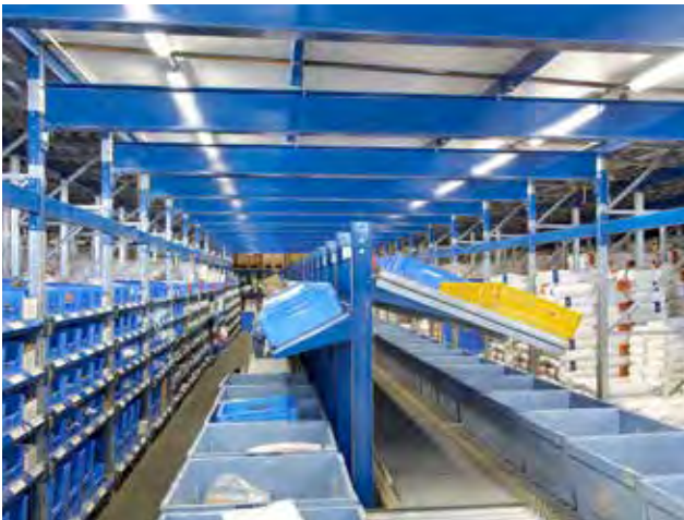
On conveyor lanes
