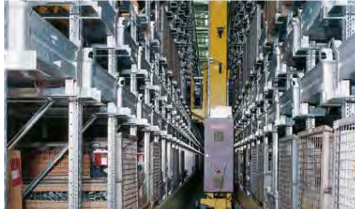
Automated pallet live storage facility with single position storage
